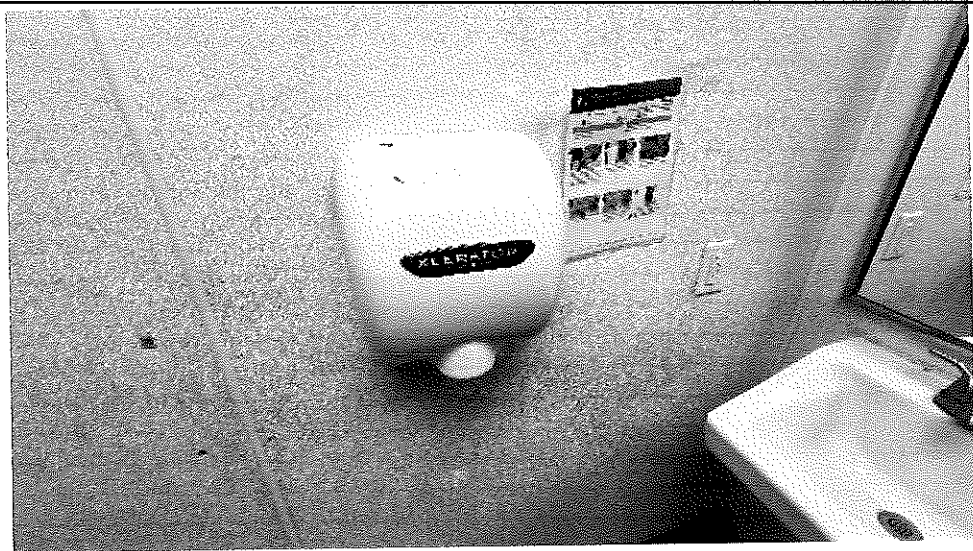
Figure 6: Excel XLERATOR / early high-speed dryer / black mold on wall
