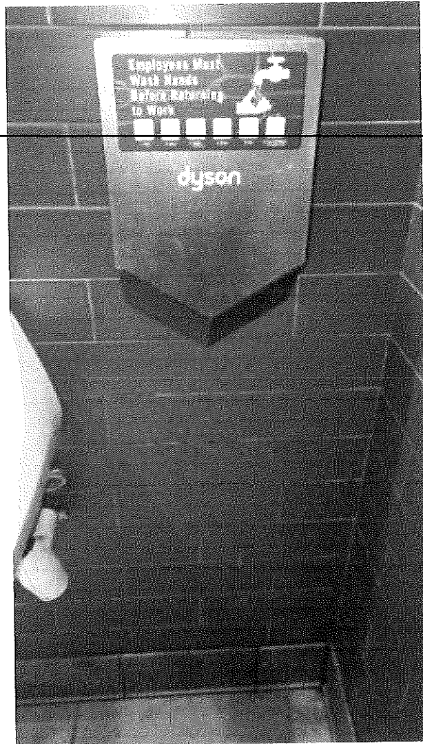
Figure 9: Downdraft-Dispersal dryer (Airblade V) / mold on wall, water staining on floor
