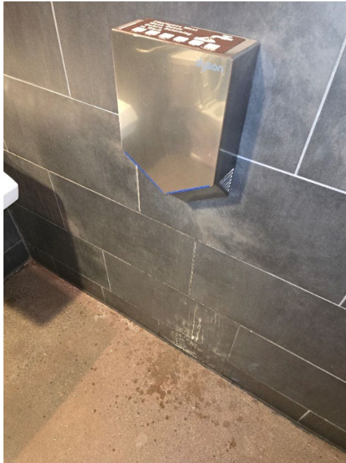
Dyson Airblade V downdraft dispersal dryer with water visible on walls and floor
